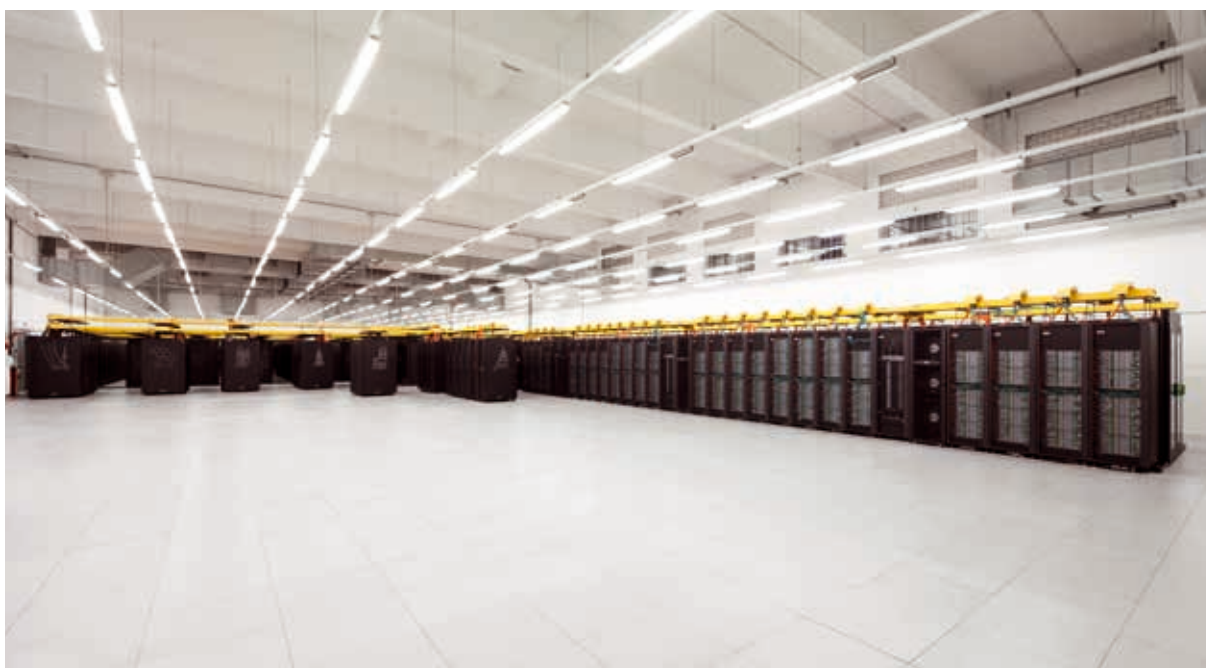
Figure 1: SuperMUC Phase 1 on the left and SuperMUC Phase 2 on the right, in the server room.
