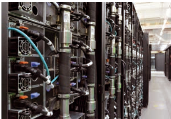
Figure 4: Rear of racks with warm water cooling.
